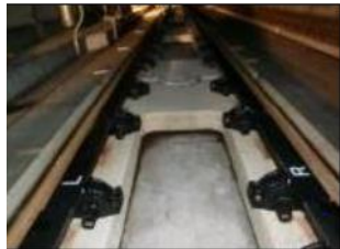
Derailment prevention guards
